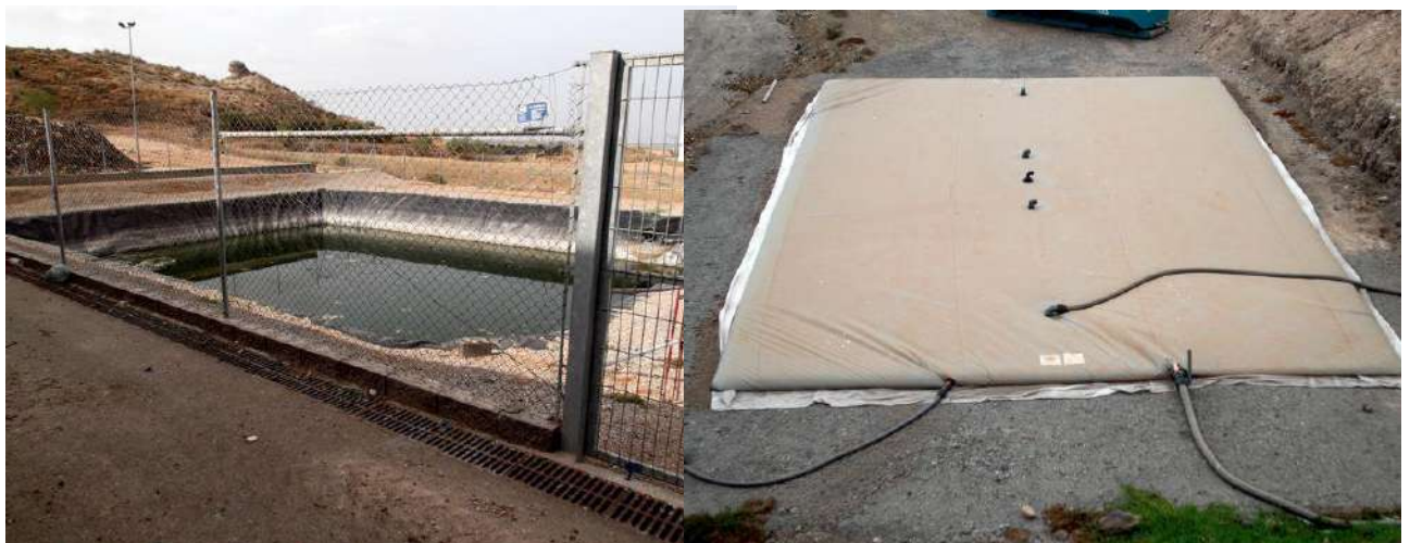
Figure 38. Examples of different leachates storage room. Left, opened tank with a perimeter fence. Right, a tank closed to avoid odour problems and the excess of rainfall.
